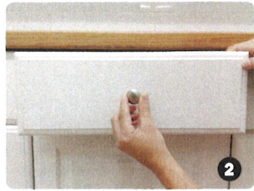
2 Place hardware (measure as needed) to find position you like; mark hole location with pencil (We are centering on width and height)
