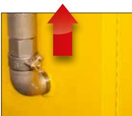
Bottom left vents chemical vapors to outdoors, away from workers.
