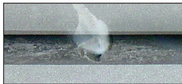
PROBLEM: Damaged A/C aluminum line
