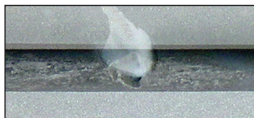
PROBLEM: Damaged A/C aluminum line
