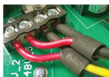
DC Wire Insulator
