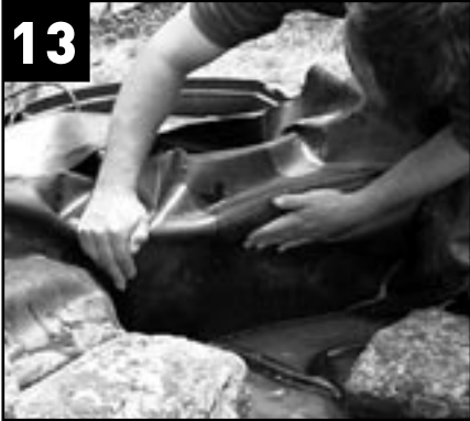
13 Position pond liner over the Skimmerfilter™ mouth and hold it in place. Smooth liner free of wrinkles and folds. Wipe clean.
